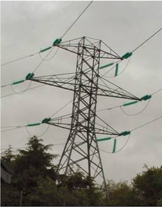
Figure 11 - Typical strain angle structure used to terminate a transmission line section.
