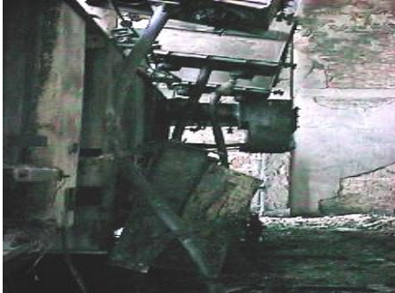
Ph. 3 Burnt out 240 MVA transformer after a 132kV cable termination failure
