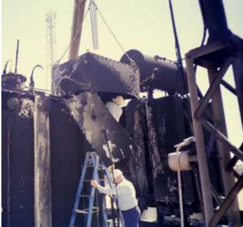
Ph 5 cable box after fire in ph.4. Cables & gland plate blasted off by arcing fault
