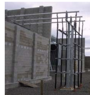
• Ph. 6 Cable terminations
