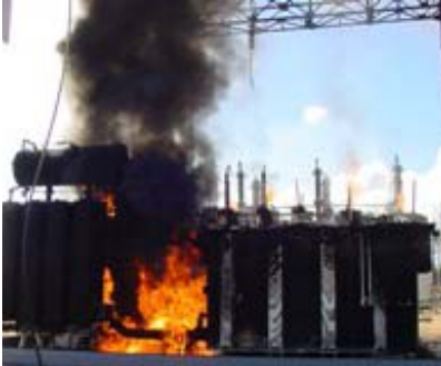
Ph. 4 Transformer fire caused by 11kV cable termination failure
