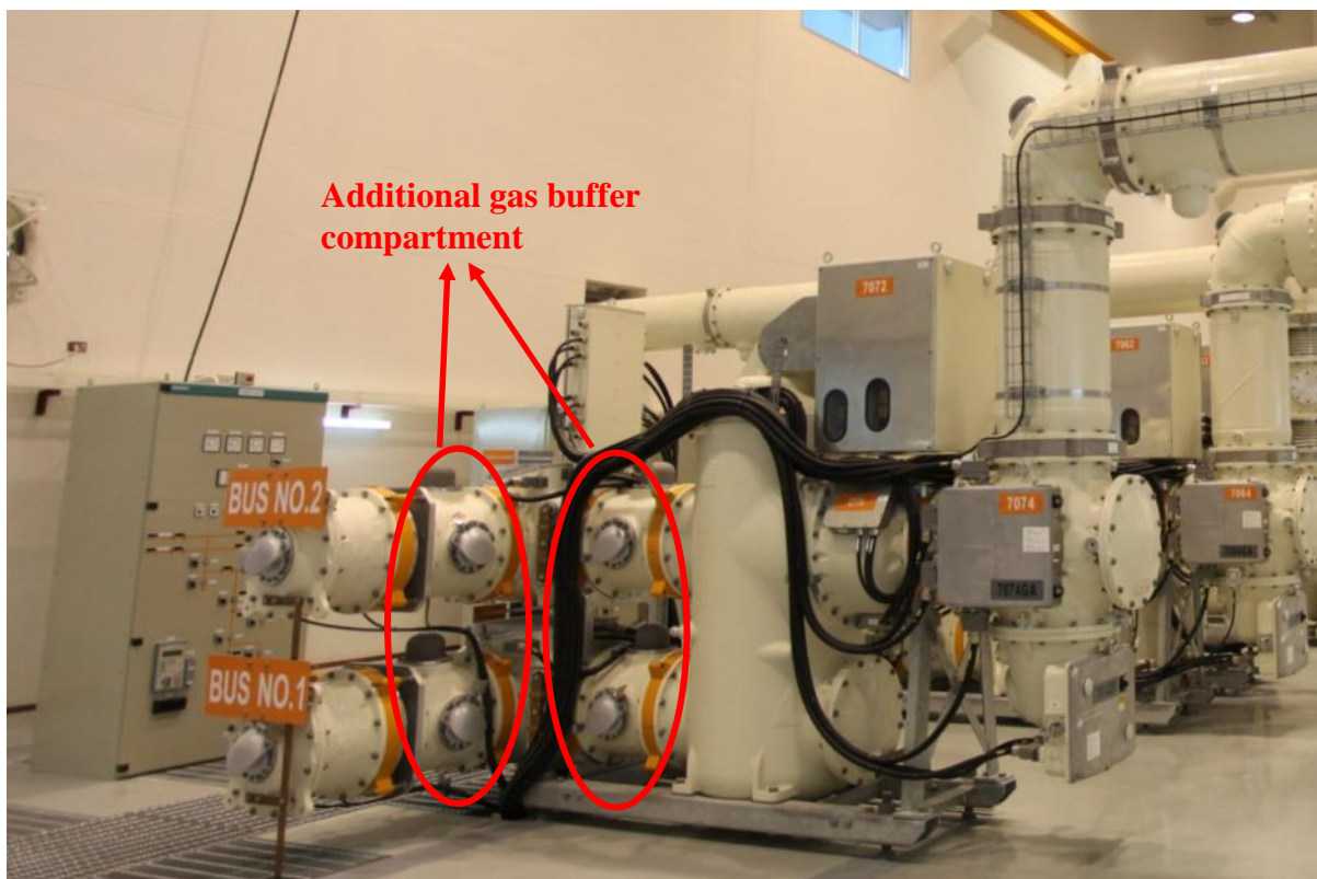
Fig.13 115kV GIS Hua Wai substation
